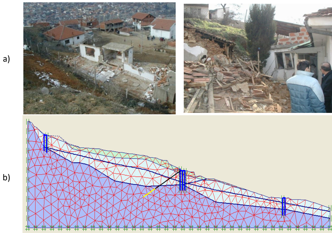
Fig. 17 (a) Some of the consequences of the last reactivation of landslide Ramina in 1999, and (b) geotechnical modelling for remediation design purposes (prepared by J Josifovski 2014).
